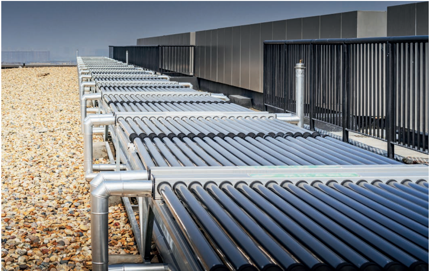
Solar water heating thermal collector system
